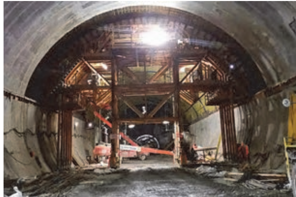
The Confederation Line’s Rideau Station under construction, part of Ottawa’s LRT project.
